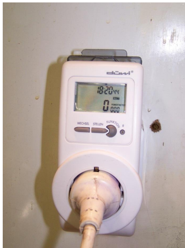
Device for measuring the useful power of the generator
